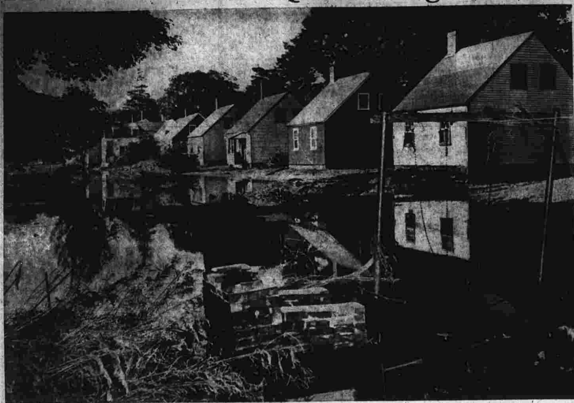
Note the water line on the roofs of these devastated homes.
